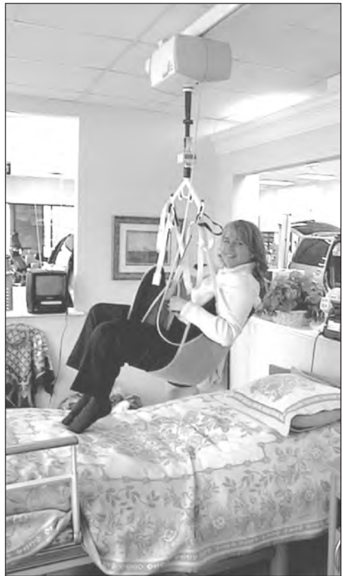
Photo 4 - Ceiling mounted powered lift with battery back-up (Photo by Jim Karl)
